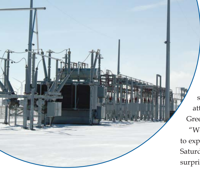
We Energies built the Blue Sky Green Field energy center's substation adjacent to ATC's substation.
